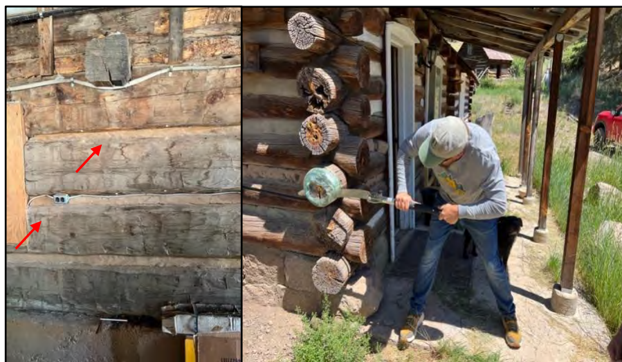
The locations of the two core samples (CDM 2 and CDM 3) on the north wall of the two-story cabin are shown here at left, and a cross section (CDM 5) on the one-story cabin at right.
