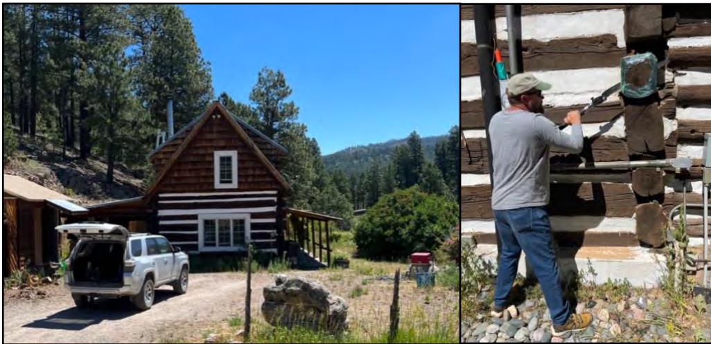
View of the west side of the two-story Casa del Mañana log cabin (at left), and cutting the log end (CDM 1) on the east side (at right).
