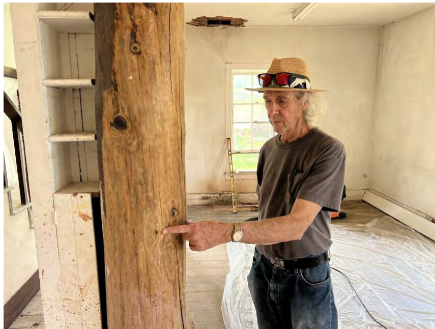
Fig. 2. The large ponderosa pine vertical support post in the living room (Adams 3). The post is set against the north wall and carries part of the upstairs floor load. Its obviously improvised position (notably, it is not structurally integrated with the masonry wall behind it) suggests that it was added during a later remodel; the tree-ring date of 1922 or 1923 confirms this.
