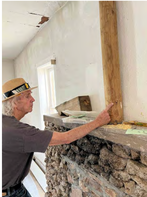
Fig. 11. Detail of the ponderosa pine post (Adams 4) extending from the fireplace mantle toward the ceiling. The outer (cutting) date of this sample is 1922, contemporary with the ponderosa pine vigas in the northeast addition.
