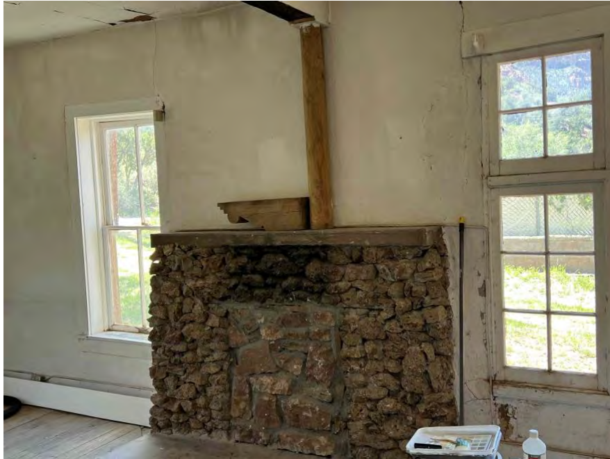
Fig. 3. The living-room fireplace, showing the smaller vertical ponderosa pine post (Adams 4) rising from the mantle toward the ceiling. The pole is somewhat oddly positioned, again suggesting post-hoc structural reinforcement rather than a feature of the original build.
