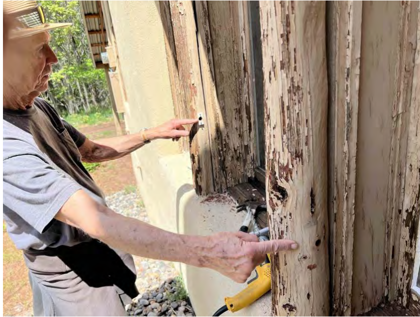
Fig. 1. Roger Sweet pointing out the two juniper window-header timbers (Adams 1 and Adams 2) in an exterior, south-facing wall. Each was cored for tree-ring analysis.
