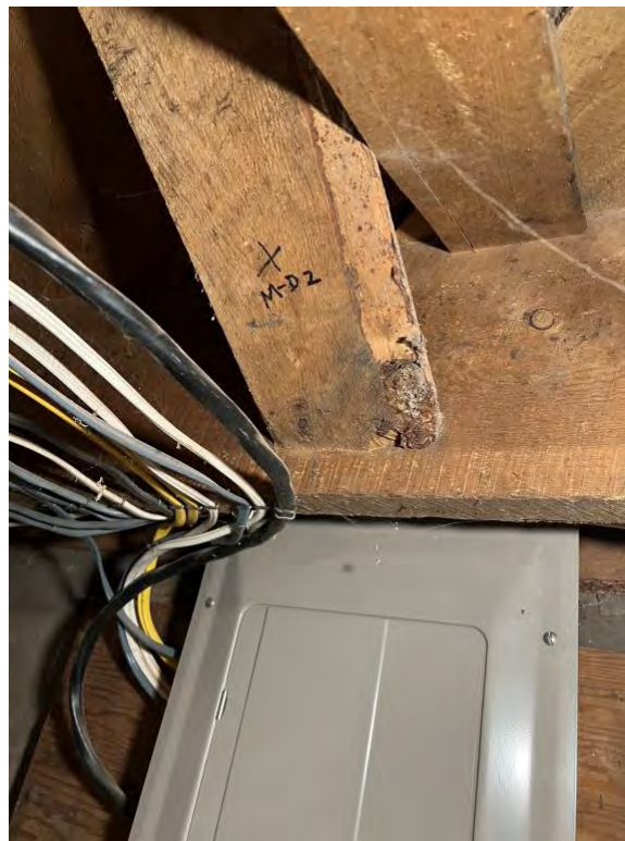
Fig. 3. Sample MD-2 in situ above the electrical circuit breaker box, before removal.
